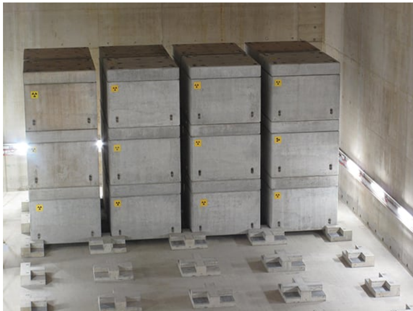
Figure 4.1-2. ILW storage at the Trawsfynydd (UK)
