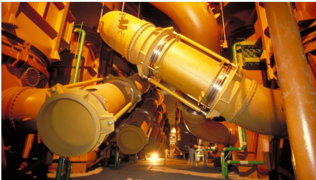
Figure 3.3.3-3. A cascade of diffusors at the Georges Besse (France) enrichment plant
